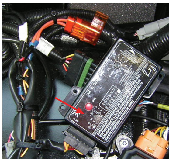
Figure 10. Electronic timer in main fuse compartment
