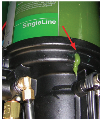
Figure 6. Unplugged overflow hole
