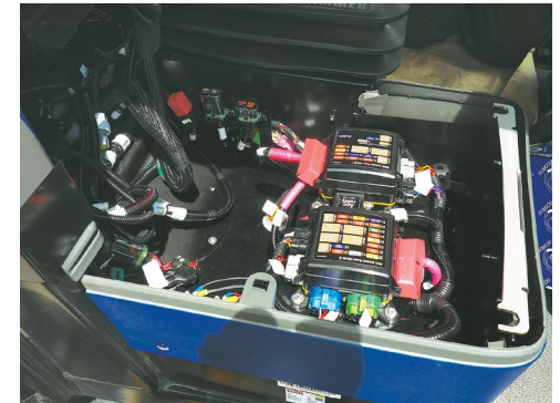
An opened electrical compartment (cover removed).
