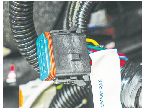
SMARTRAX connector in the electrical compartment.
