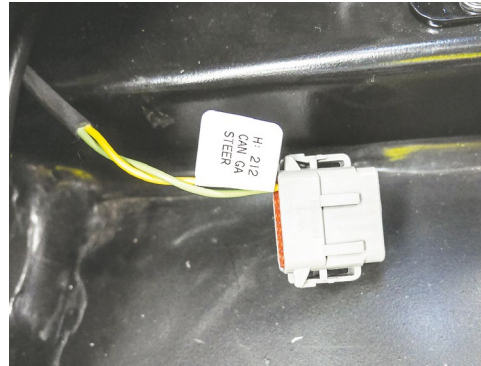
Steering CAN connector in the electrical compartment.
