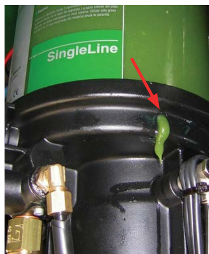
Unplugged overflow hole
